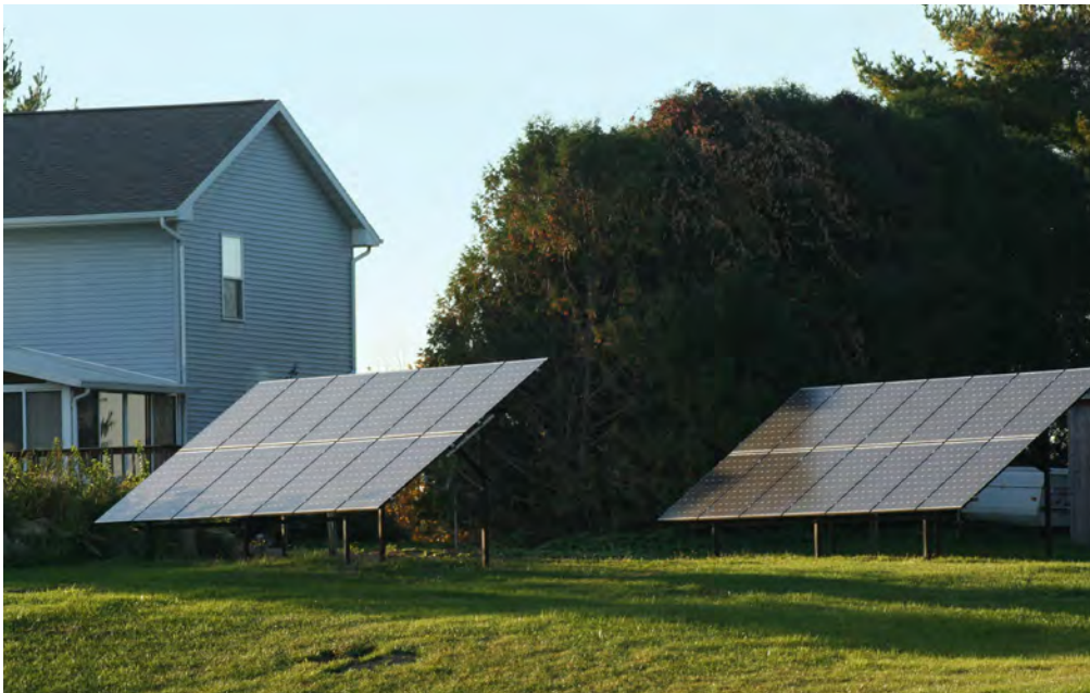
▲ Panels impacted by tree shading.
