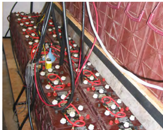
▲ A battery bank
